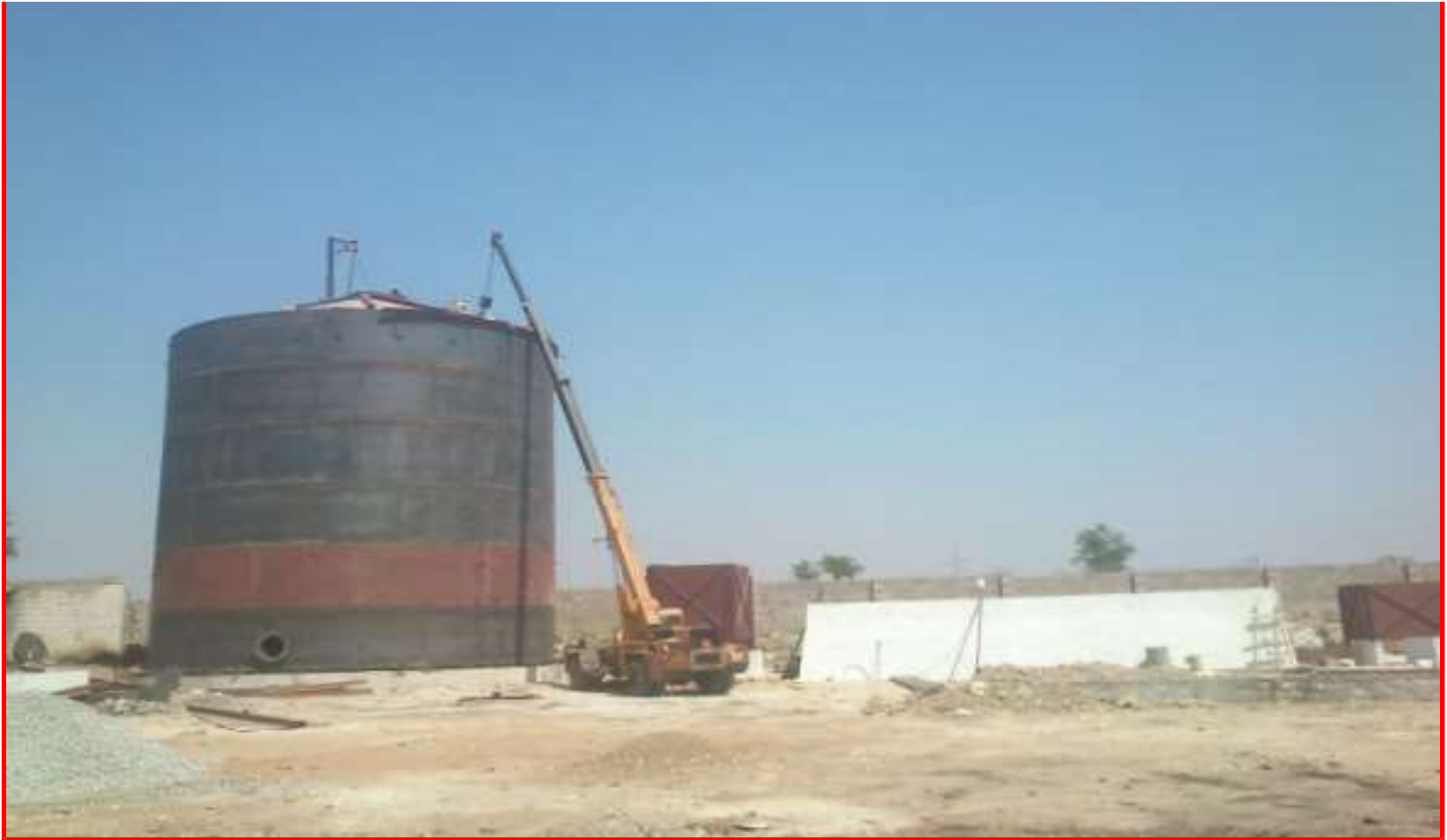
Anaerobic Reactor Shell-2
