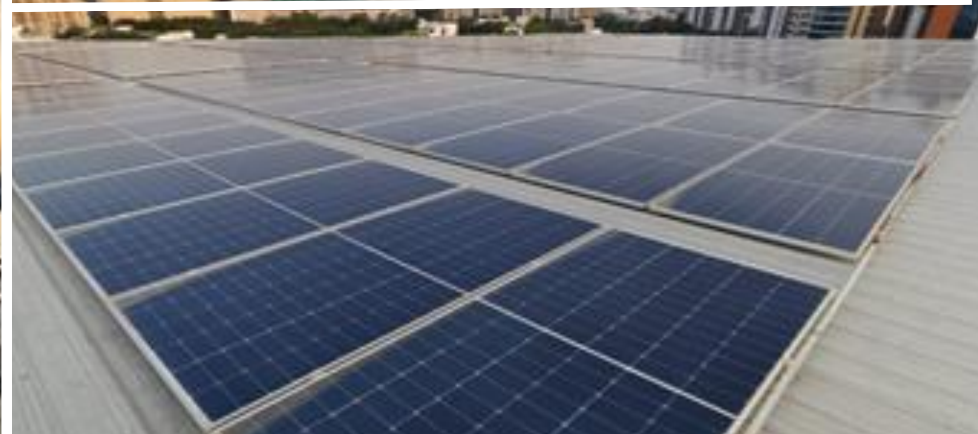
100 % Roof Space Utilization for Solar Power Generation
