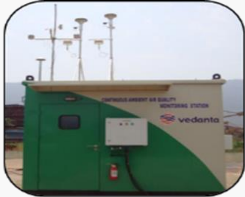
Continuous Ambient Air Quality Monitoring Station (CAAQMS)
