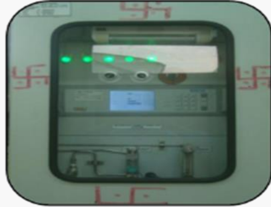
CEMS at Power Plant
