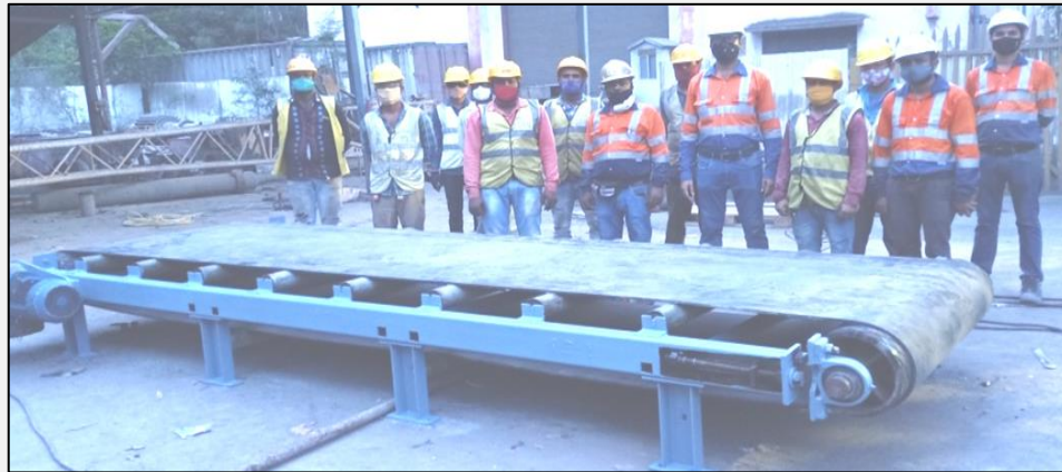
Conversion of Screw of Multiplex to Belt conveyor
