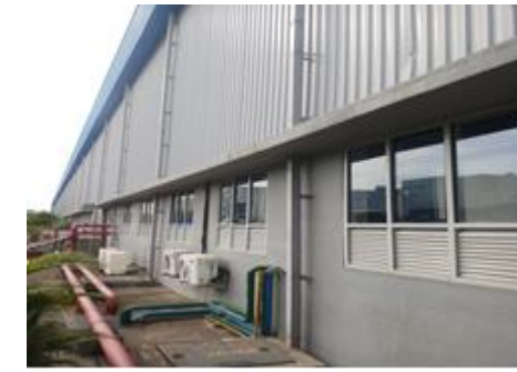
100% Roof area covered in Rainwater harvesting
