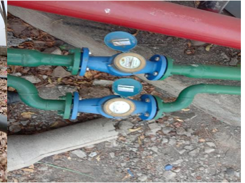
Water Meters for monitoring
