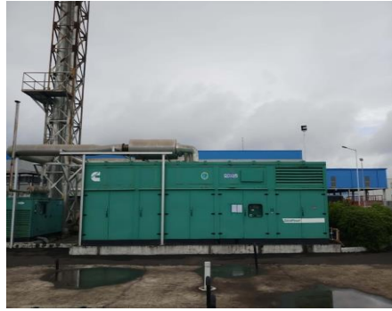
Energy efficient DG sets
