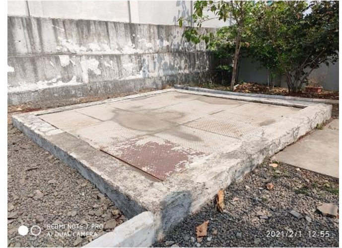
Rainwater harvesting tanks
