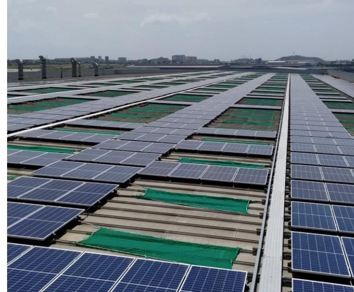
Roof top solar panels
