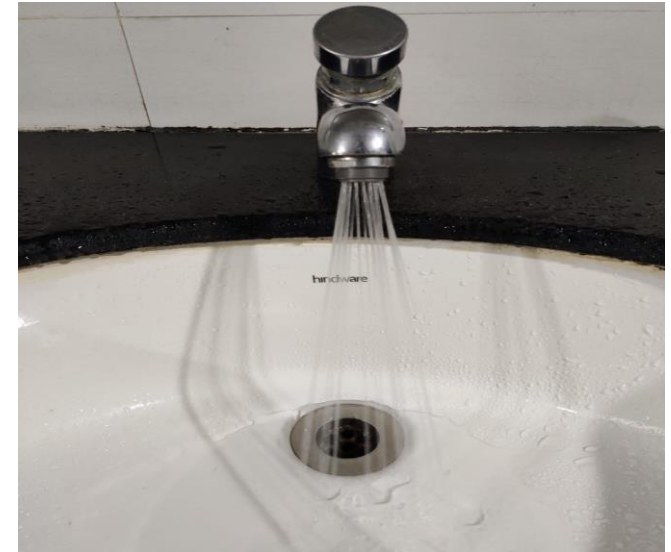
Water saving taps
