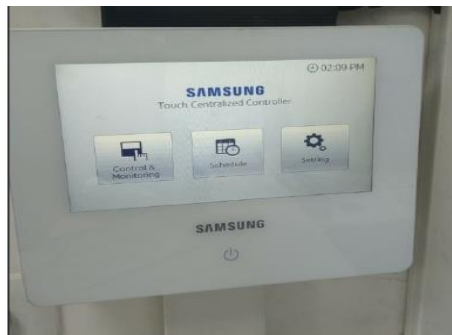
AC unit controller system
