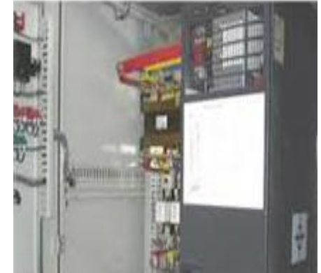
VFD for paint shop blowers
