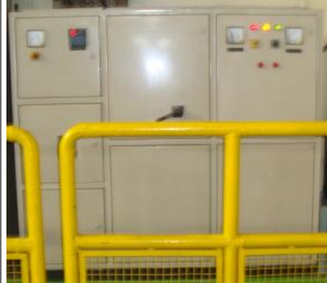
Voltage regulators for lights
