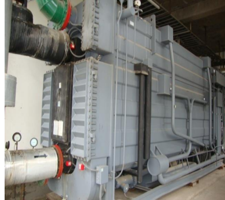
VAM for Plant Air Conditioning
