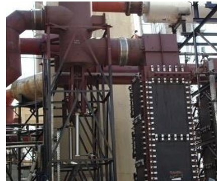
Waste heat Recovery unit (HRU)
