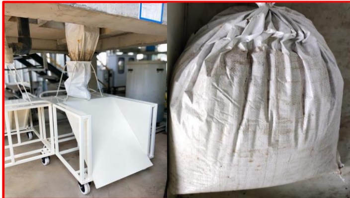
Sludge processing & handling
