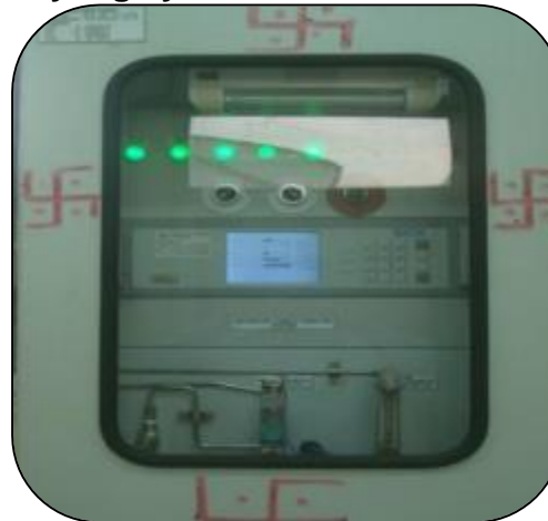
CEMS at Power Plant
