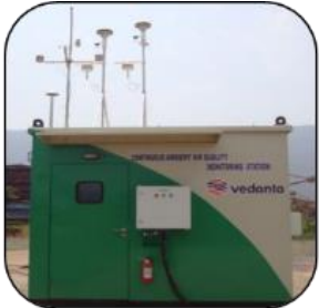
Continuous Ambient Air Quality Monitoring Station (CAAQMS)
