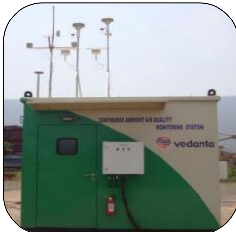
Continuous Ambient Air Quality Monitoring Station (CAAQMS)
