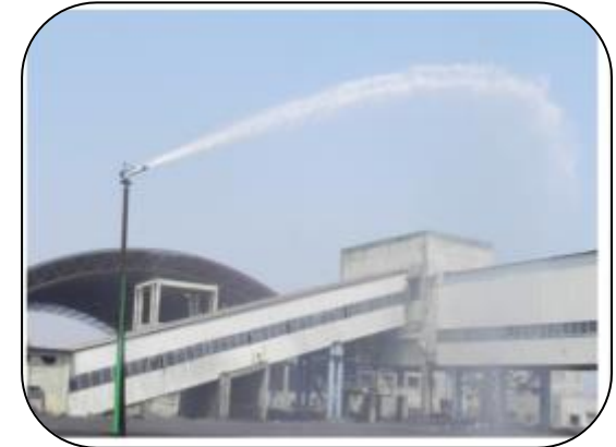
Water sprinklers at Coal handling
