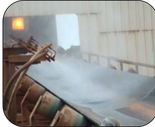
Dry fog system at bauxite handling
