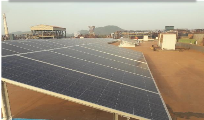
Solar Power Station in HR Bldg.
