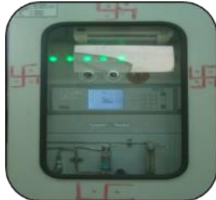
CEMS at Power Plant
