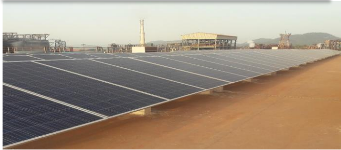
Solar Power Station in Adm. Bldg.
