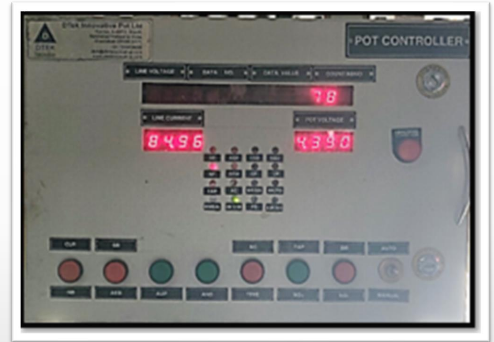
PLC controller installed at pot
