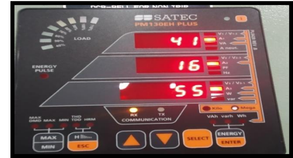
Integrated Energy Meters
