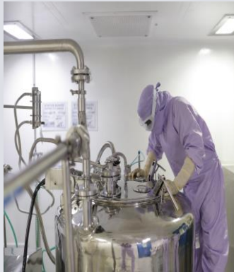
Additional Clean Room Facility, Bidar
