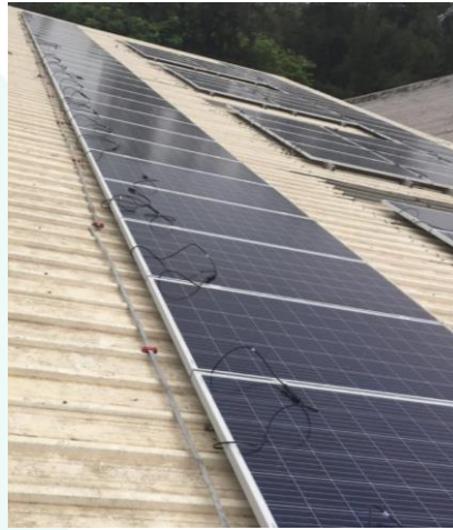
Solar PV Panels
