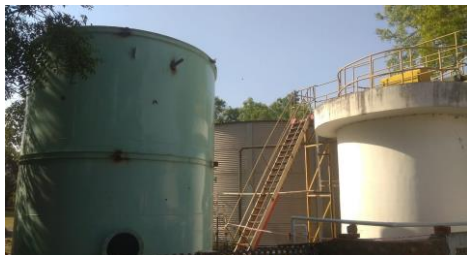
Municipal STP treated water plant – 50 kLD
