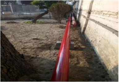
Overground fire hydrant system
