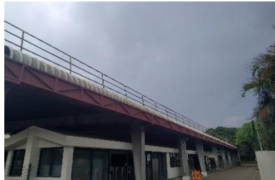
Roof edge protection system
