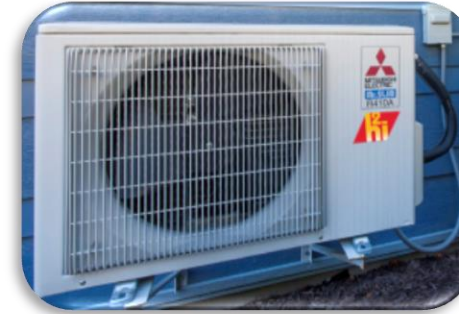
EE air conditioning
