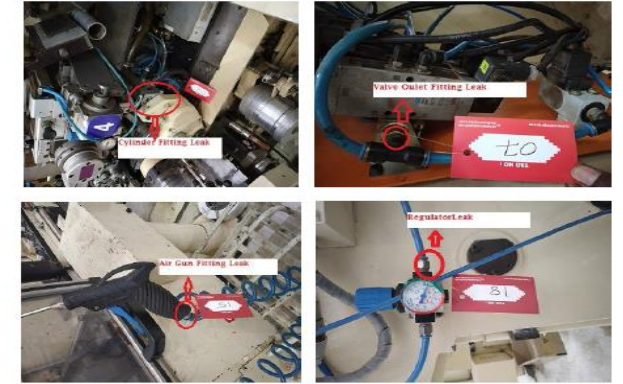
Compressed Air Audit
