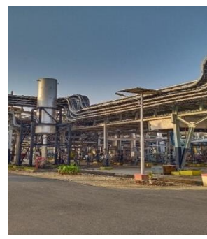
Solar Unit at Plant
