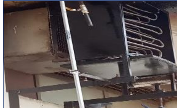
Heat Recovery system in Stem dryer exhaust
