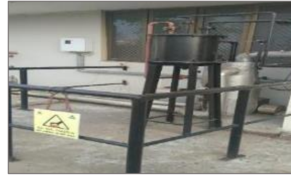
Cylinder condensate recovery (2% improvement in condensate recovery)
