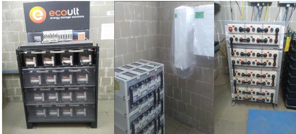
Battery Testing Lab
